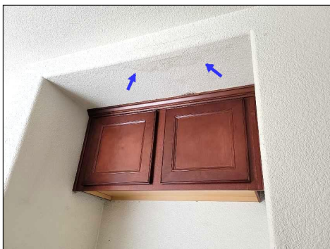
Past water damage
