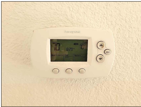
Down stairs Thermostat
