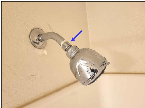
Shower head leak upstairs guest
