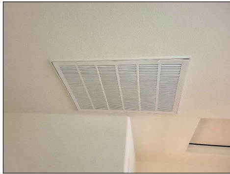
Filter up stairs hall ceiling
