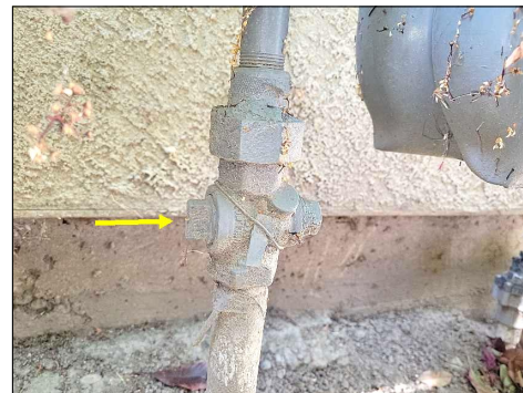
Main gas shut off valve
