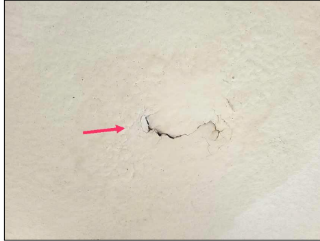
Past water damaged to ceiling in flex room
