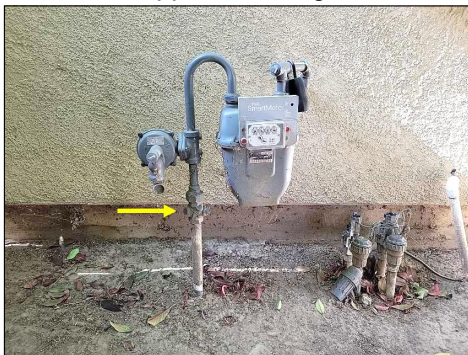
Main gas shut off valve
