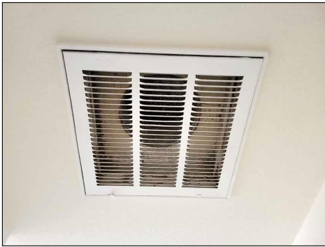
Filter is missing
