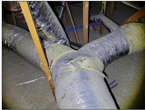
View of ducting
