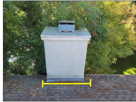
No cricket flashing present
