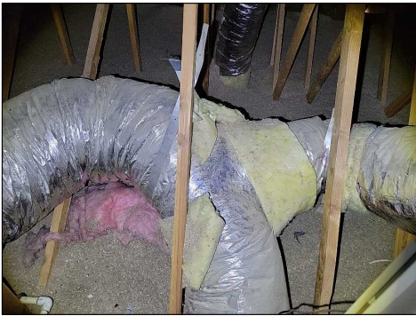
View of ducting
