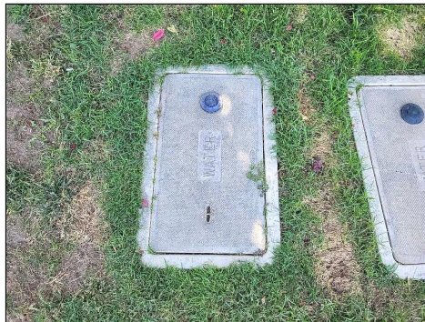
City water access at the sidewalk
