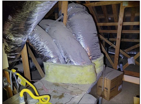
View of ducting
