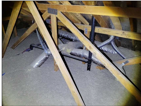
View of ducting
