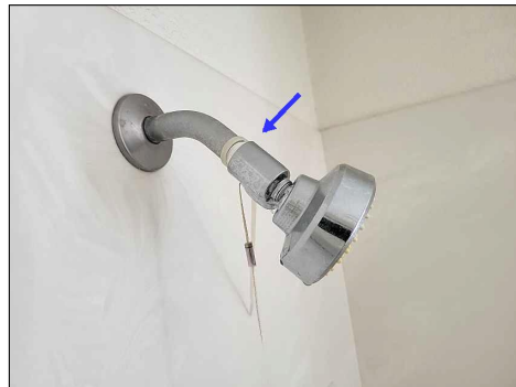
Shower head leak primary
