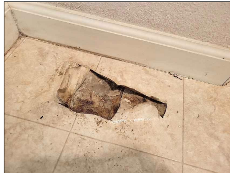
Damage to flooring
