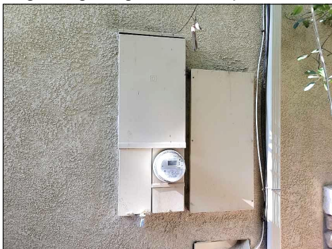
Main electric panel
