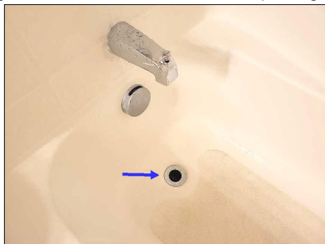
Tub stopper was missing upstairs guest
