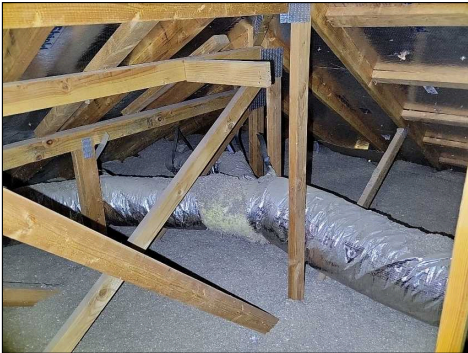
View of ducting
