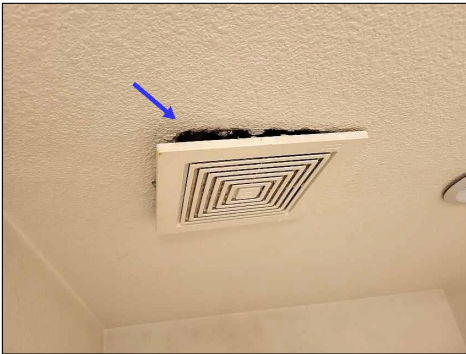
Up stairs bath fan is loose
