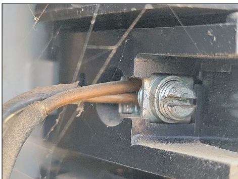
Double tap wiring
