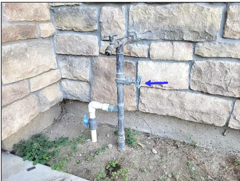
Main water shut off valve
