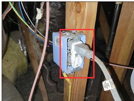
Outlet cover missing
