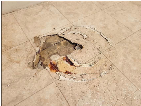
Damage to flooring
