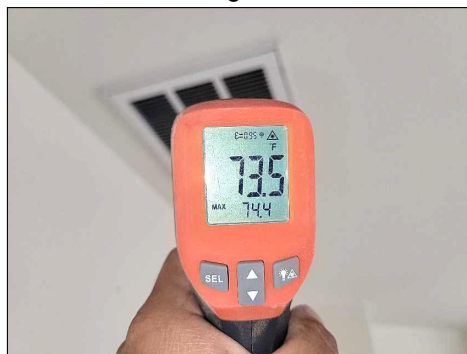
Return temp primary room
